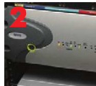
AVID DS NITRIS BOX For all the functions the Nitris box enables Neal to perform, it takes up surprisingly little rack space.
