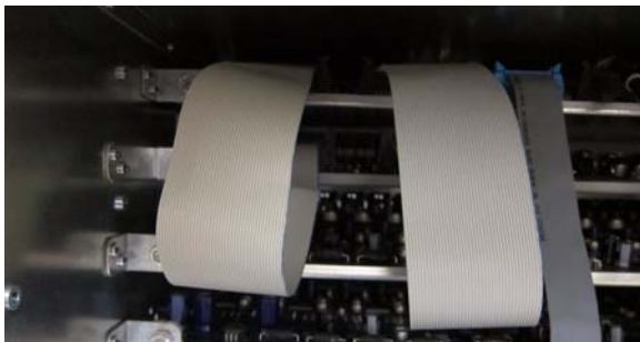
IOx ribbon cables connected to FOH IO card
