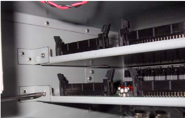
Securing the IOx card to the FOH Rack chassis
